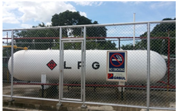
Above ground tank inside secure compound
