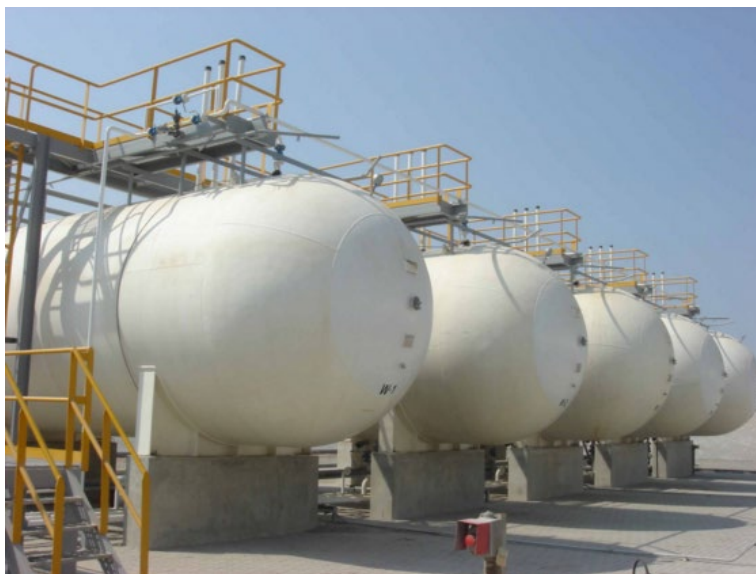
An example of a Bulk LPG facility
