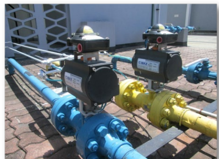
Emergency shut down valves
