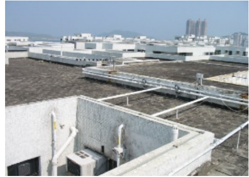
Ring main on top of a multistorey apartment block
