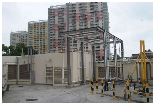
Parking bay for bulk LPG road tanker with fire-fighting facilities
