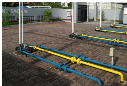
Tank fittings clustered onto a single manifold
