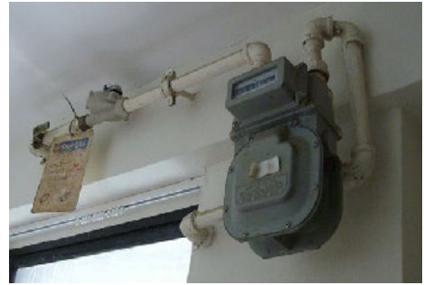
LPG meter installed inside an apartment
