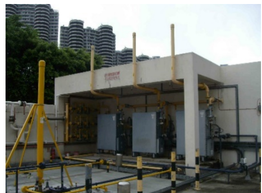
Underground LPG tanks and vapouriser room
