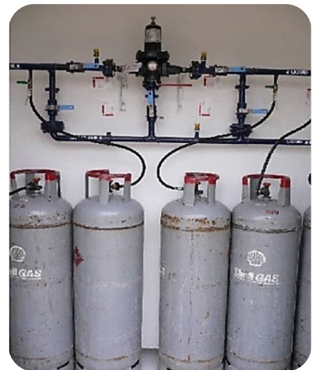
Small multi-cylinder LPG storage facility
