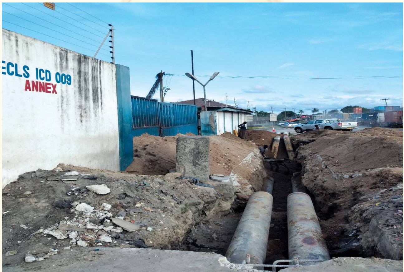
Figure 33: Exposed underground pipelines crossing ICD entrance gate at Kitopeni area in Dar es Salaam.
